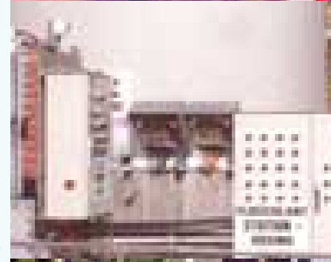
Flocculant blending and dosing equipment
