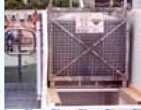
Bunding and chemical dosing
