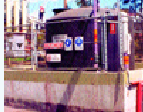
Bulk chemical storage
