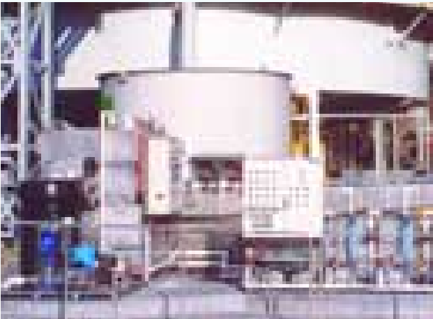
PBT1000 unit with multiple dosing pumps installed at a mine site NSW
